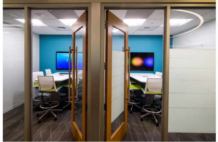
GENISYS A2 Troffers were installed in meeting rooms & collaboration areas.
